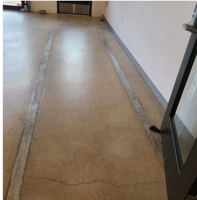
Floor Slab Cracking
